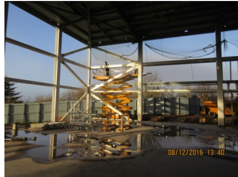
Photograph 6 Steel erector carrying out paint remediation. When the steel is chained for lifting into position the paint protection is "rubbed" off. The paint is reapplied when the steel is in situ.
