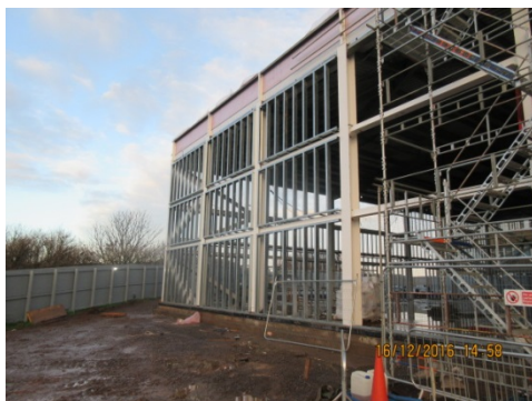
Photograph 11 Following completion of main structural steelwork the steel erector has now commenced the erection of the external steel partition frame. First works on the sports hall.
