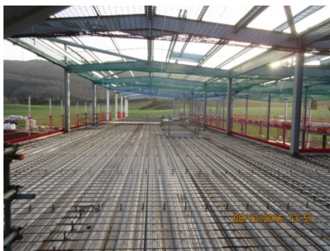
Photograph 3 Reinforcing installed to 1st and 2nd floor up to grid point M
