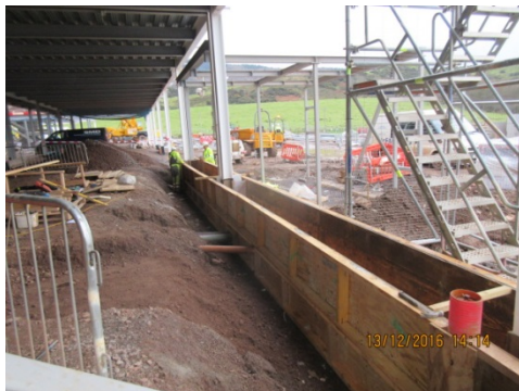
Photograph 9 Perimeter formwork shutter being installed for the ground floor slab between grid point E and J(1)
