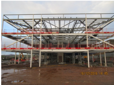
Photograph 7 – The South gable end of the new school building. This marks the completion of the structural steelwork.
